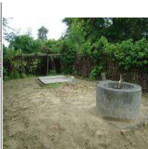
Fig: Biogas Digester in Operation
