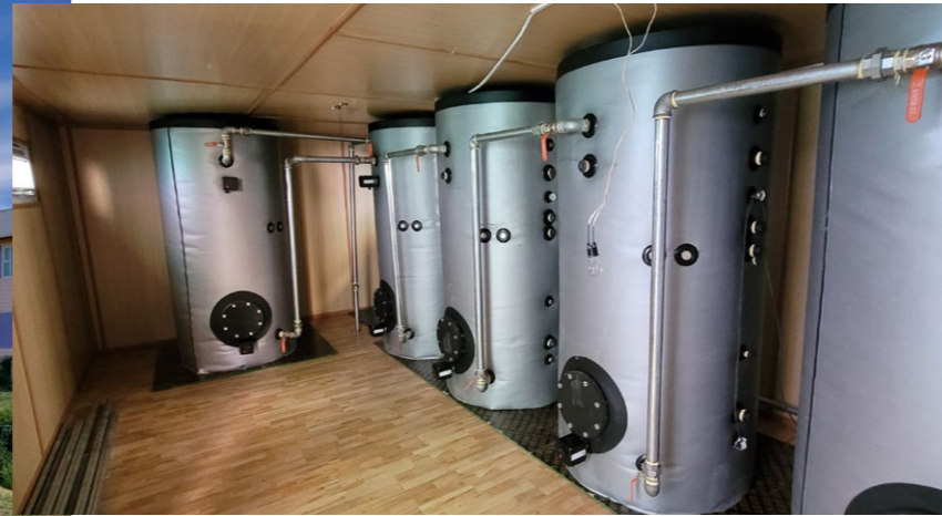
Latent heat accumulators in Mongolia store heat for long periods and release it when needed
