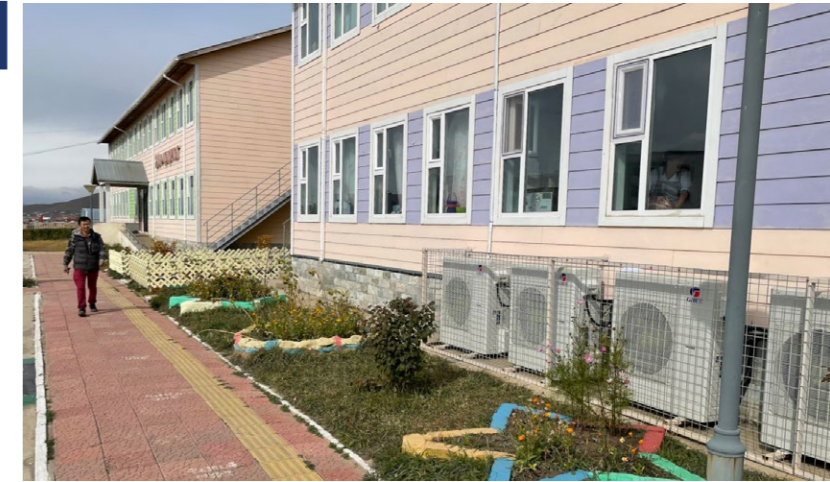
Efficient air-to-air heatpumps heat this school even at outside temperatures of -40 °C.
